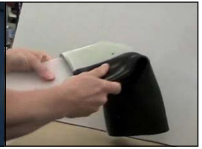
Liner is rolled over a piece of plastic to pre-stretch the liner and create a flat working surface.
